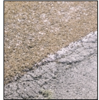
A thin application of LWA shows oil around the particles next to the exposed edge of the old deteriorated road surface.
