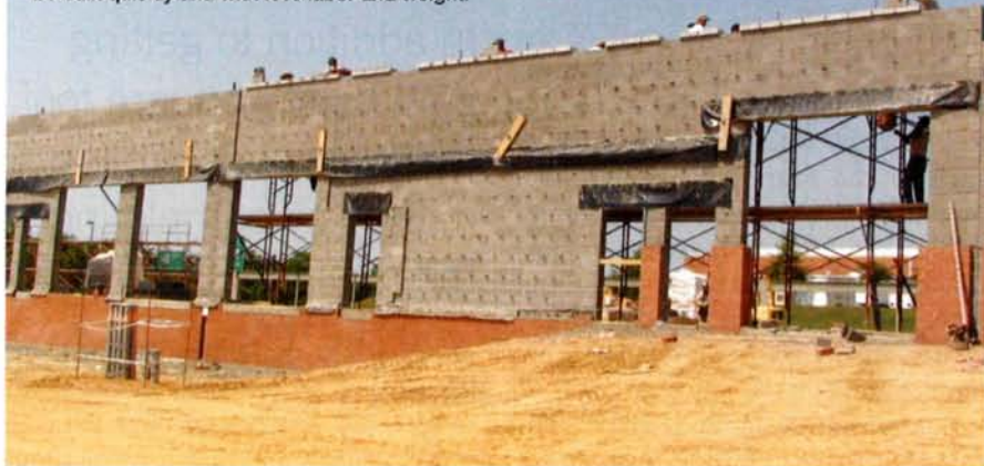
Lightweight masonry units allowed the six new warehouses at the Maryland Science Center in Baltimore to be built quickly and with less labor and weight.
