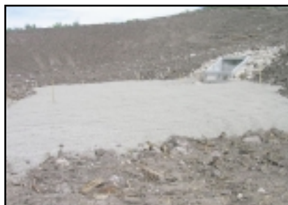
Photo I.D. Underground filter fill
