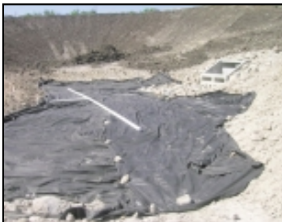
Photo I.D. Underground filter fill
